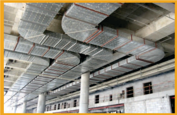
Modular Cleanroom HVAC / Ducting
